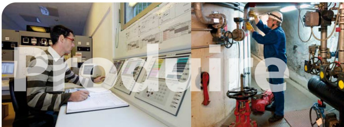
Figure 90 : Revin hydroelectric power plant
