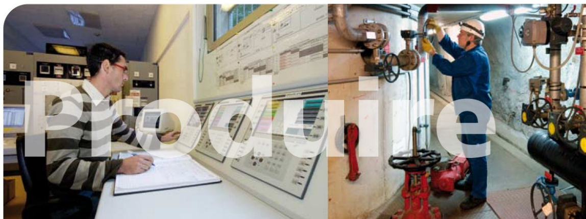
Figure 90 : Revin hydroelectric power plant
